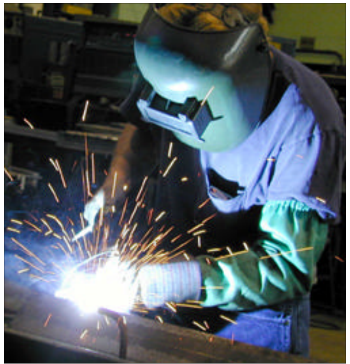
Cutting steel: At South Main, Lee Soucie tackles a fabrication job, cutting angle iron for use in a mixer wash pit at one of the company’s concrete plants
