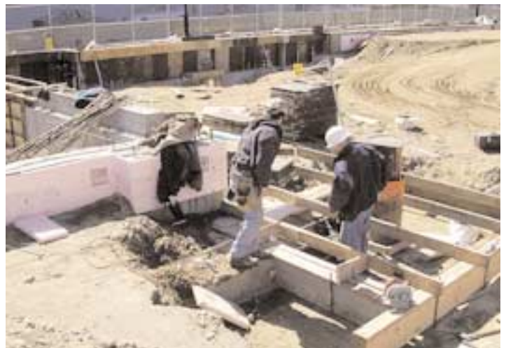
UConn at Storrs and at Waterbury: (top to bottom) Architect’s model of the 116,000 SF Information Technology Engineering Building that O&G is constructing for the University; mild temperatures permitted O&G to get ahead on site and concrete work for the elevator and underground auditorium (foreground) as structural steel for the building is erected; shirt-sleeves were in order in early March when concrete was poured at Storrs; in Waterbury, site and concrete work proceed in the elements without special covers or heating.
