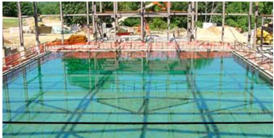
Hotchkiss School gets a new natatorium: In Lakeville, CT, O&G crews are building Hotchkiss' new indoor swimming pool. (top) Workers frame in the structure, seen to the left; (bottom) the concrete pool in the middle of its three-day water test for structural integrity.
